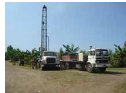
Figure 1-3: One of the public fountains in the Village of GUERIN (Leogane - HAITI); The public fountain in the Market Place - MONTRUIS - HAITI; Drilling operations in Petit Paradis (Leogane - HAITI).
