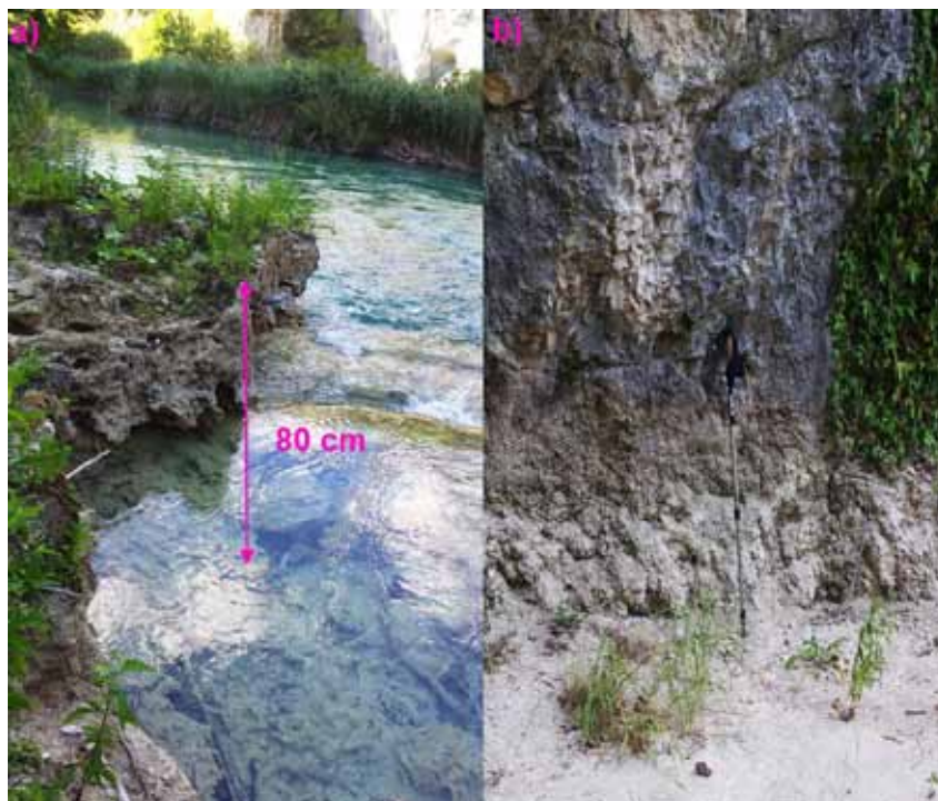
Figure 9: a) Damage at the barrier caused by anthropogenic impact in November 2011, b) Desiccation caused by damaging the tufa barriers, July 2012.
